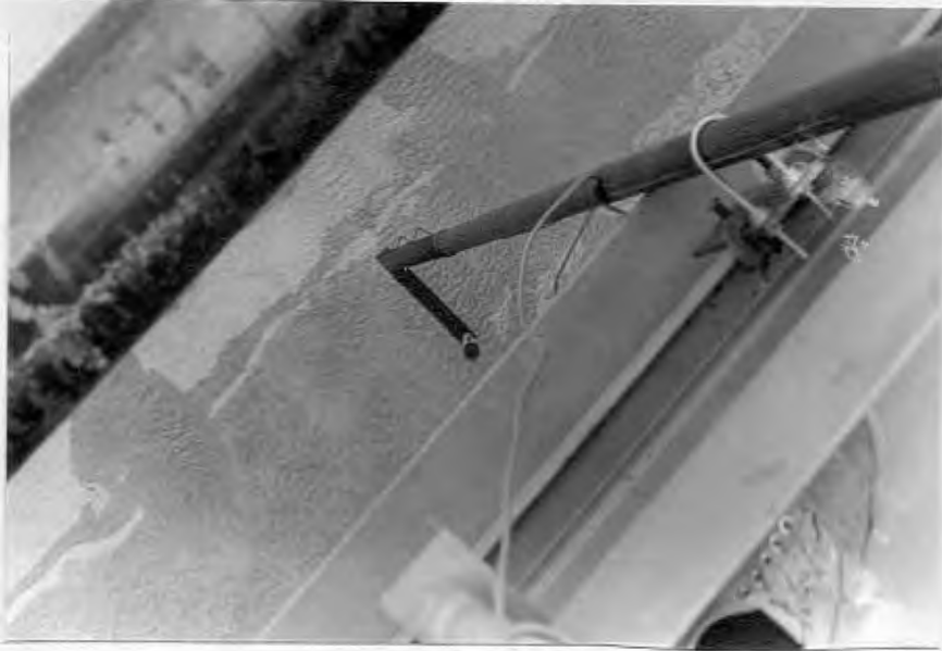
The transducer and bracket installed at the field site
