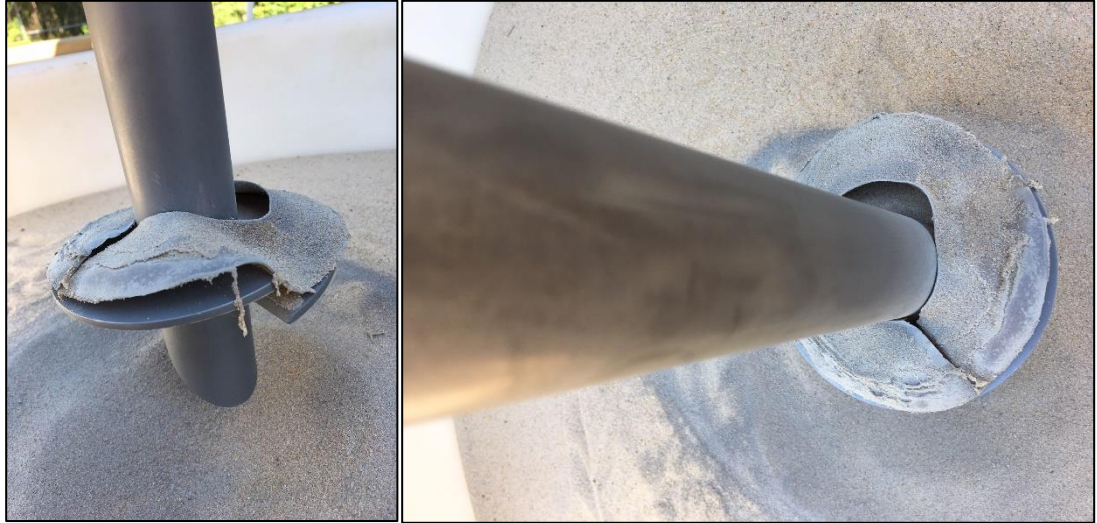
Figure 29 – Damaged Teflon sheet on anchor DSC1 after pullout
