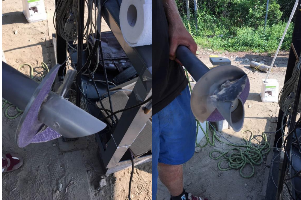
Figure 28 – Damaged sand paper on anchor DRC1 after installation and pullout
