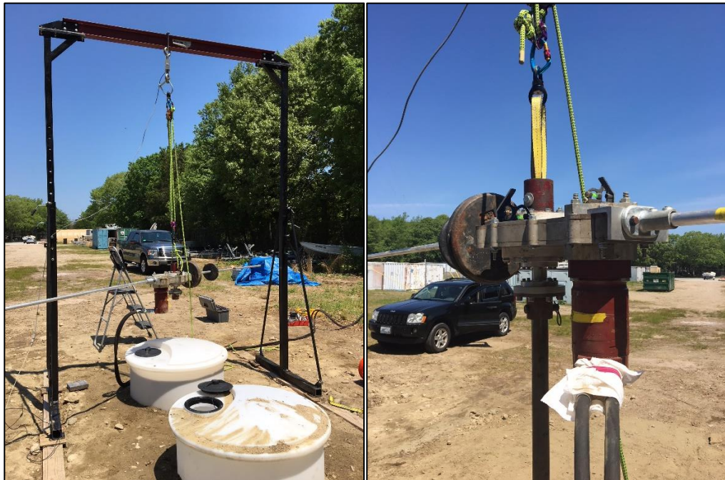
Figure 13 – Photograph of the driver system in installation setup without (a) and with anchor (b)
