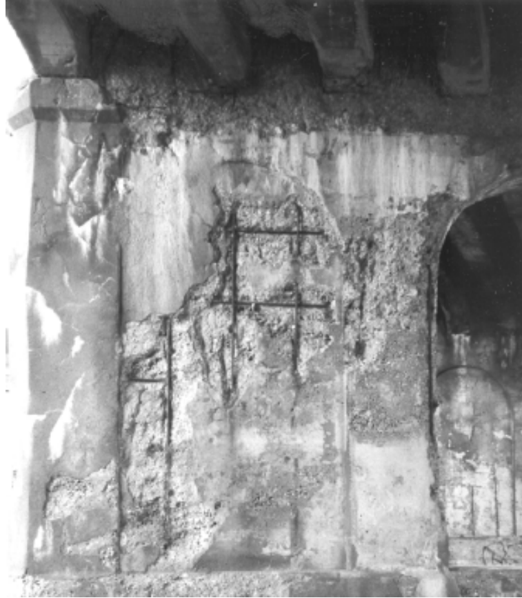
Picture 2: Severe spalling at bridge pier (Gaal 2004)
