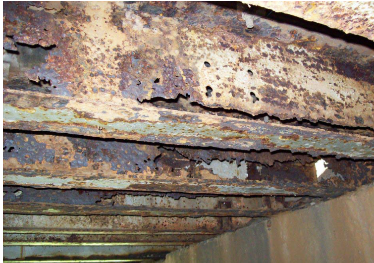
Picture 7: Steel corrosion and complete section loss on girder webs (Ryan, Thomas W. et al. 2012)
