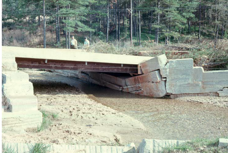
Picture 1: Abutment with undermining due to scour (Ryan, Thomas W. et al. 2012)
