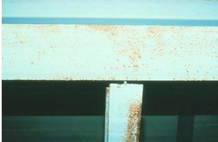
Picture 5: Pinpoint rusting at pinholes (Ryan, Thomas W. et al. 2012)
