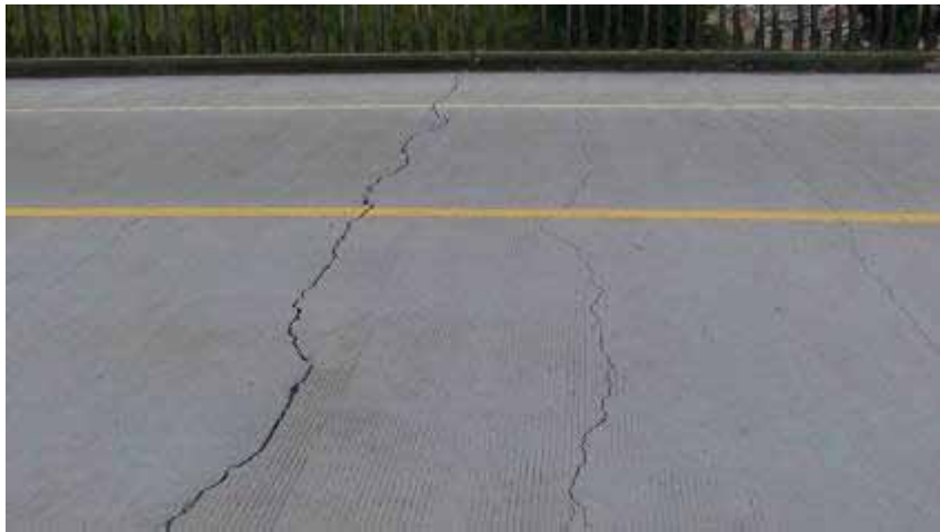
Figure 5.4: A view of Transverse Cracking on Pavement Surface
