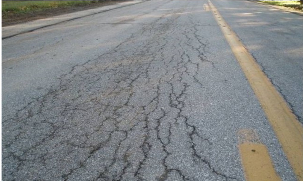
Figure 5.2: A View of Alligator Cracking on Pavement Surface
