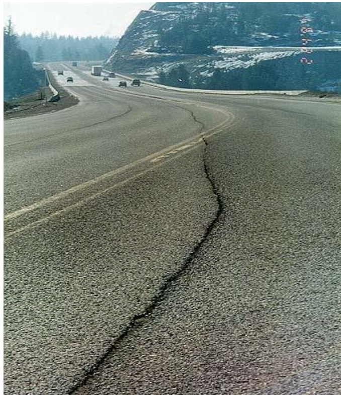
Figure 5.3: A View of Longitudinal Cracking on Pavement Surface
