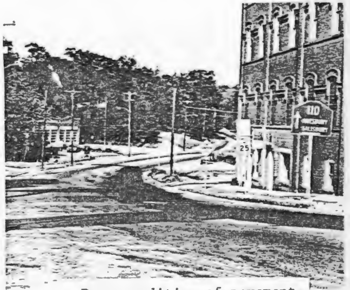
Poor condition of pavement.
