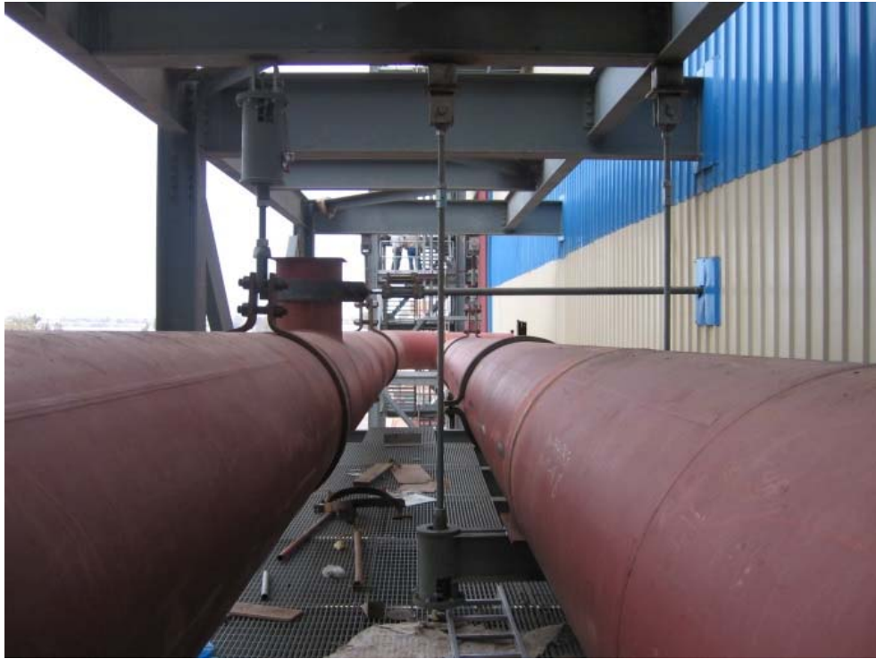
Figure 1 - Typical Pipe Support Assemblies at Sidi Krir Combined Cycle plant Alexandria, Egypt. Note the snubber in the background orthogonal to the run pipe. Palmer, Matt 2010
