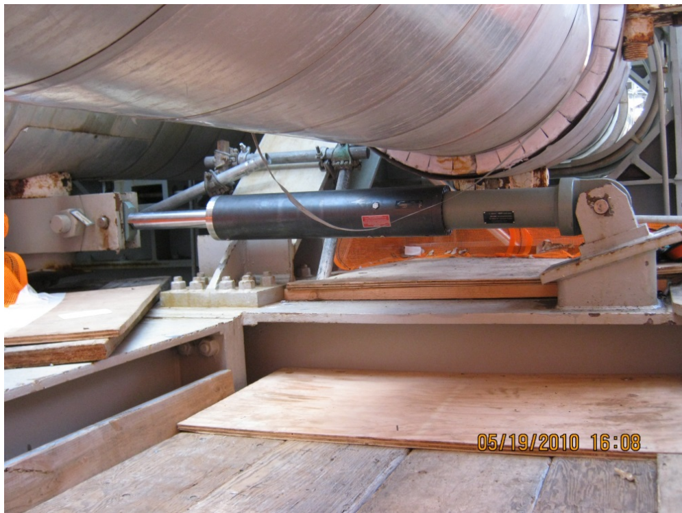
Figure 3 – Snubber installation at Diablo Canyon Nuclear Power Plant. Kewalramani, Mohan “Support 414-414BSL”. 2010
