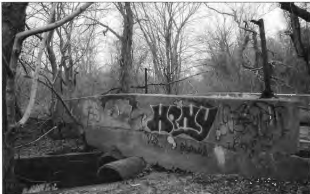
Graffiti covered bridge at the trailhead and canoe put-in on the Pawtuxet River behind Rhodes-on-the-Pawtuxet, 2002
