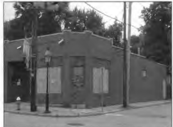
This early 20 th century commercial building in the Village core burned more than four years ago. The building was recently purchased and the new owner plans to rehabilitate it.
