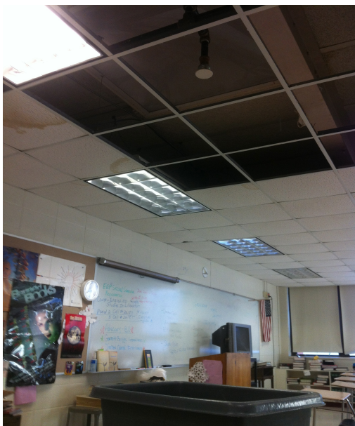
Figure 3. Rain inside the traditional classroom space Spring 2013
