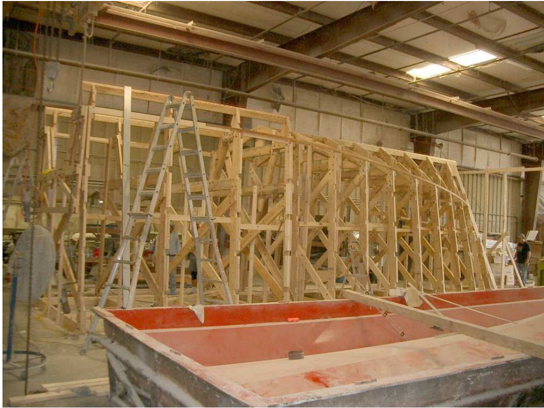
Figure A.21. Fore end of the wooden frame (i.e., plug) for building a demihull of the Gladius (center), and aft end of the mold (bottom).
