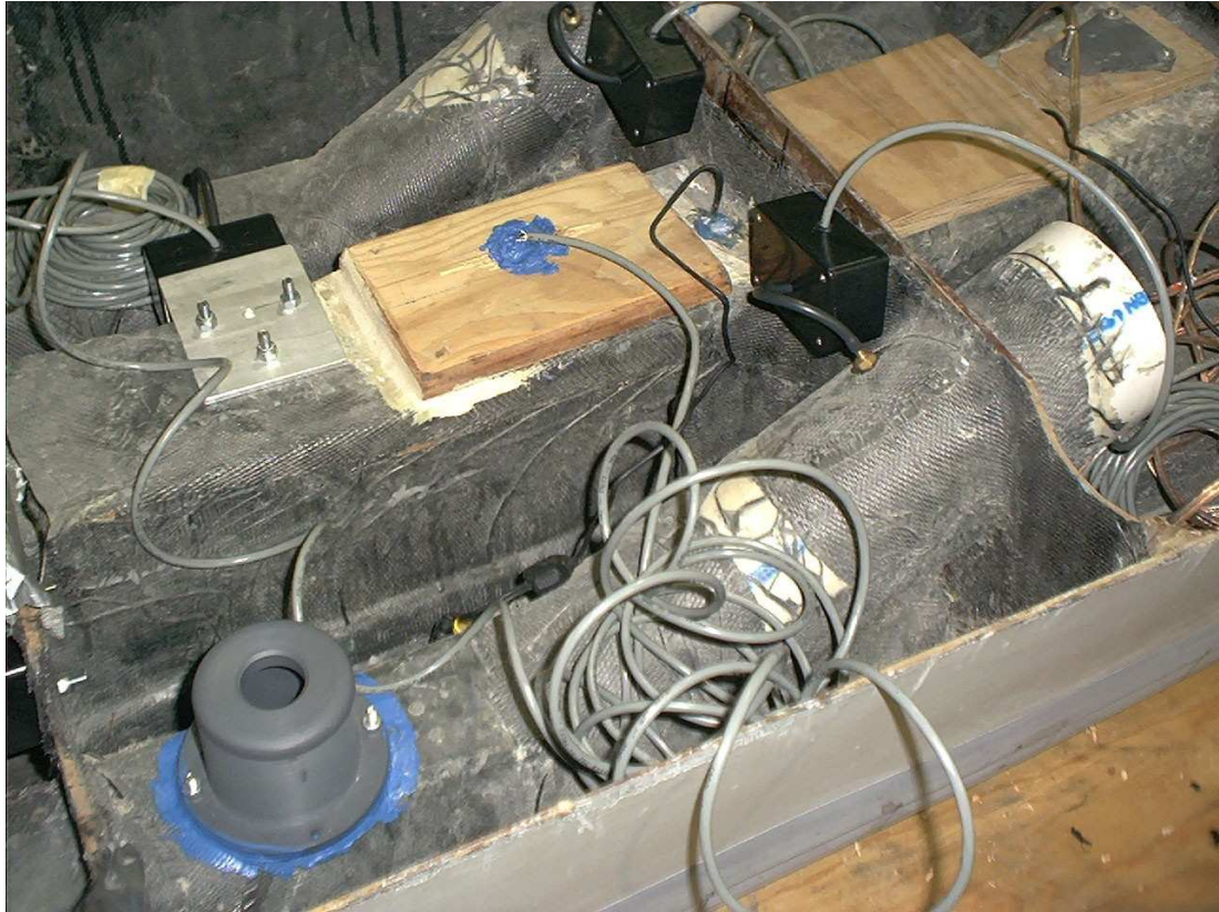
Figure A.8. View of the sensor setup of the 2.3 m model, including pressure sensors P_1 , P_2 , P_c , as well as the installation point for the range finder (bottom left). Note the air cushion inlets are not attached to ducting (top right).
