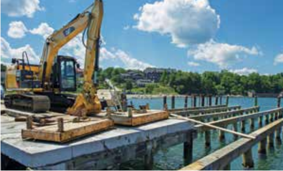
The R/V Endeavor Pier underwent major upgrades to repair damage caused by Hurricane Sandy. Photo: Alex DiCiccio
