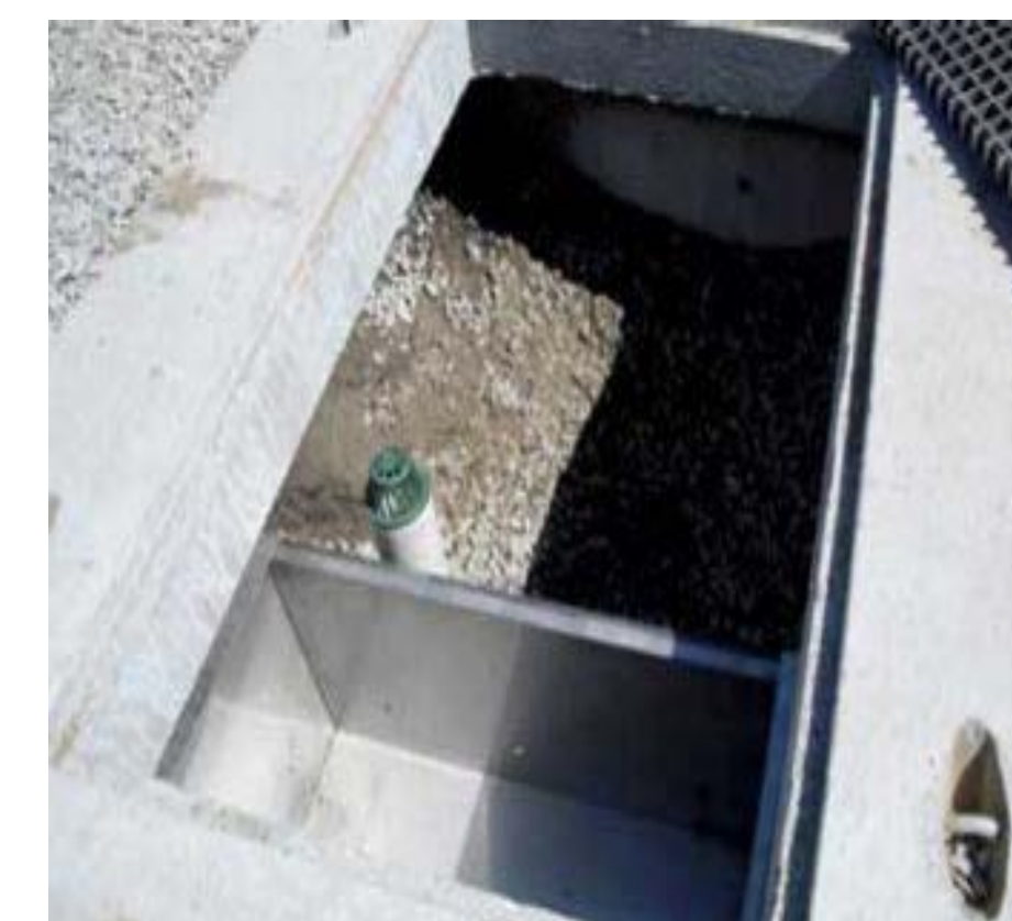
Figure 8: Interior of tree filter system ready for tree planting. In foreground, "pre-treatment" sump with weep holes; bypass/overflow pipe also shown.
