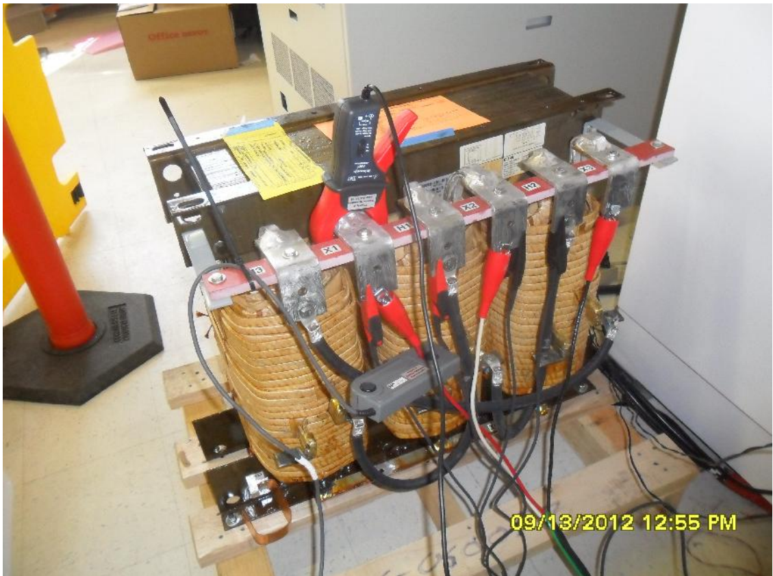
Figure 1.34: Snap picture of a 3-Phase 100KVA Transformer under test.
